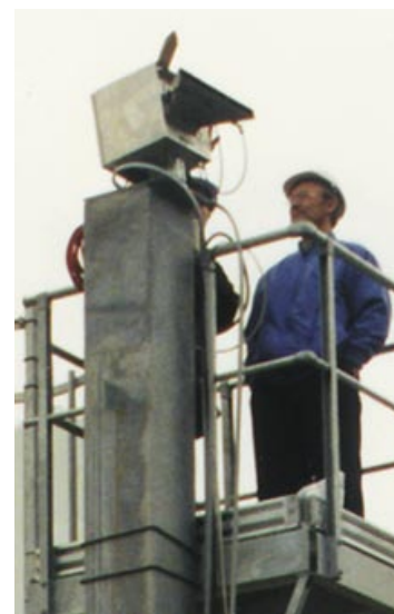
Linescanner in protective housing is mounted on top of a tower.
